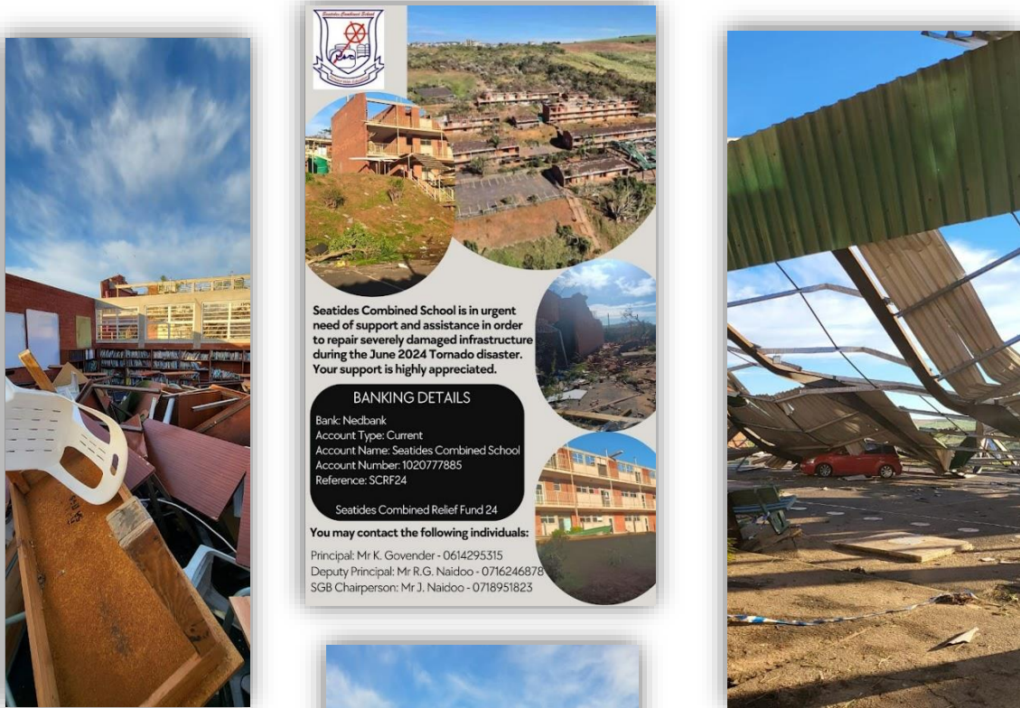
Some images of the incredible damage to Seatides Combined School.
